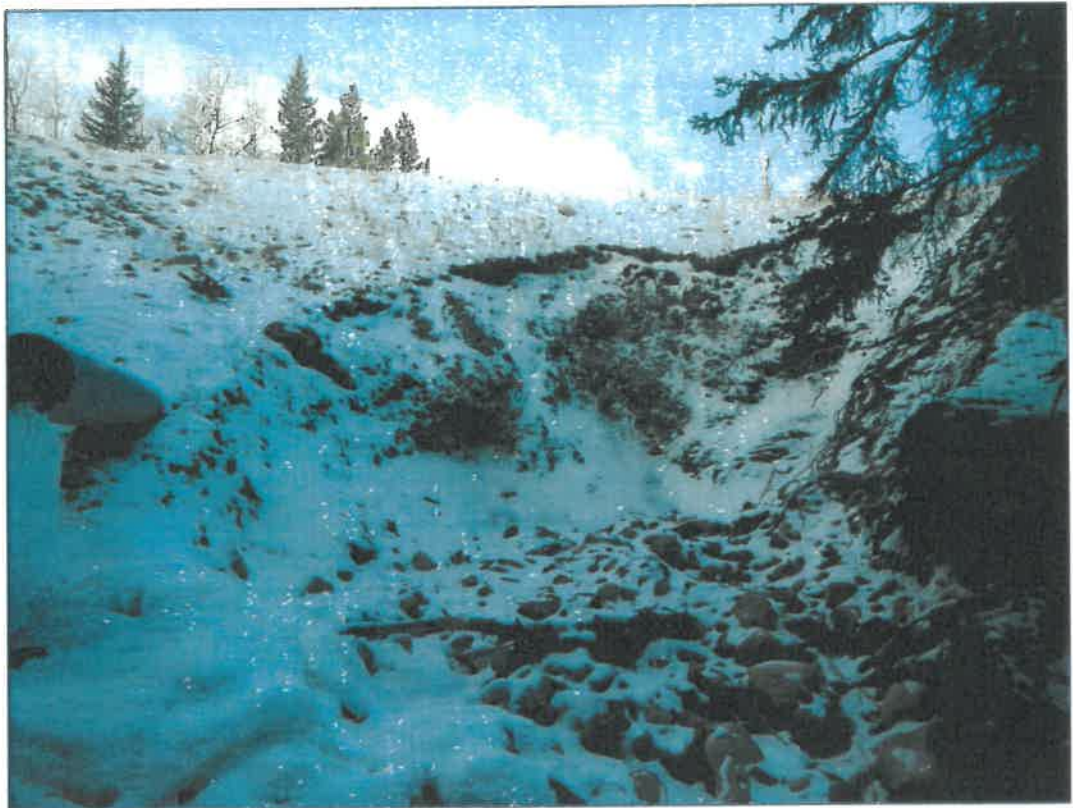
View of scour and erosion on embankment.
