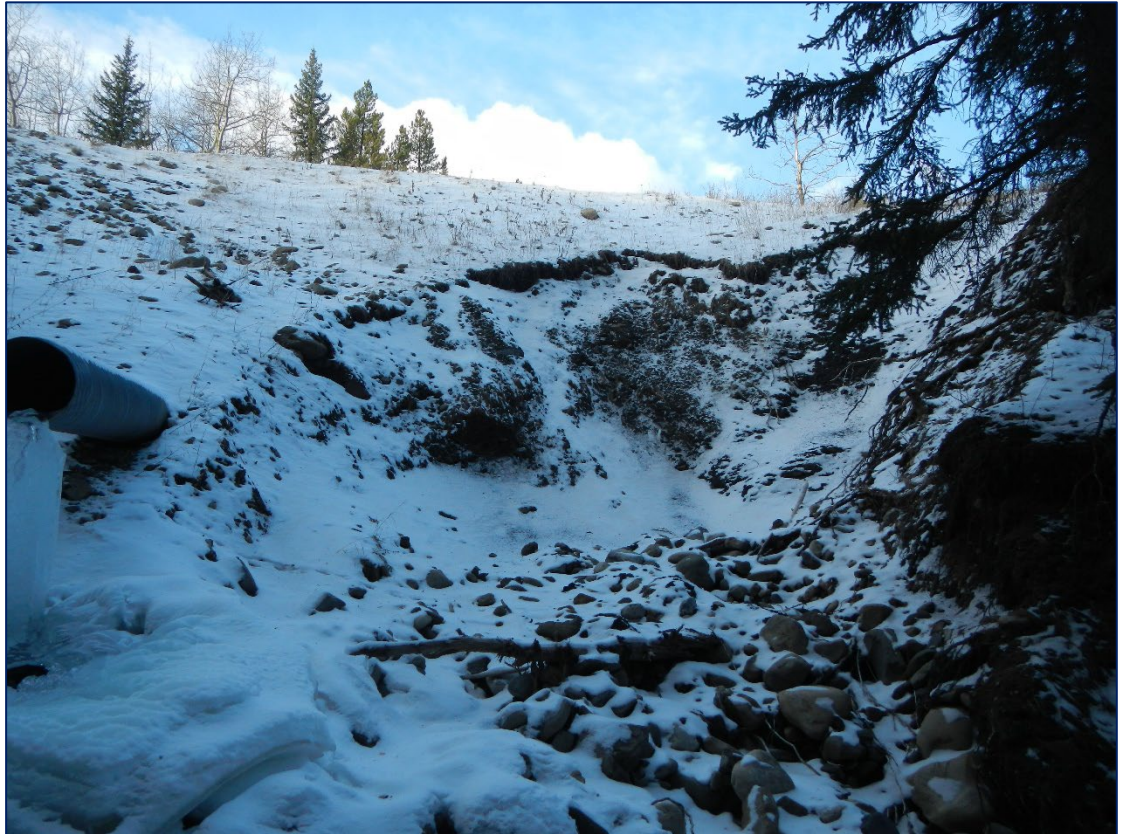
View of scour and erosion on embankment.
