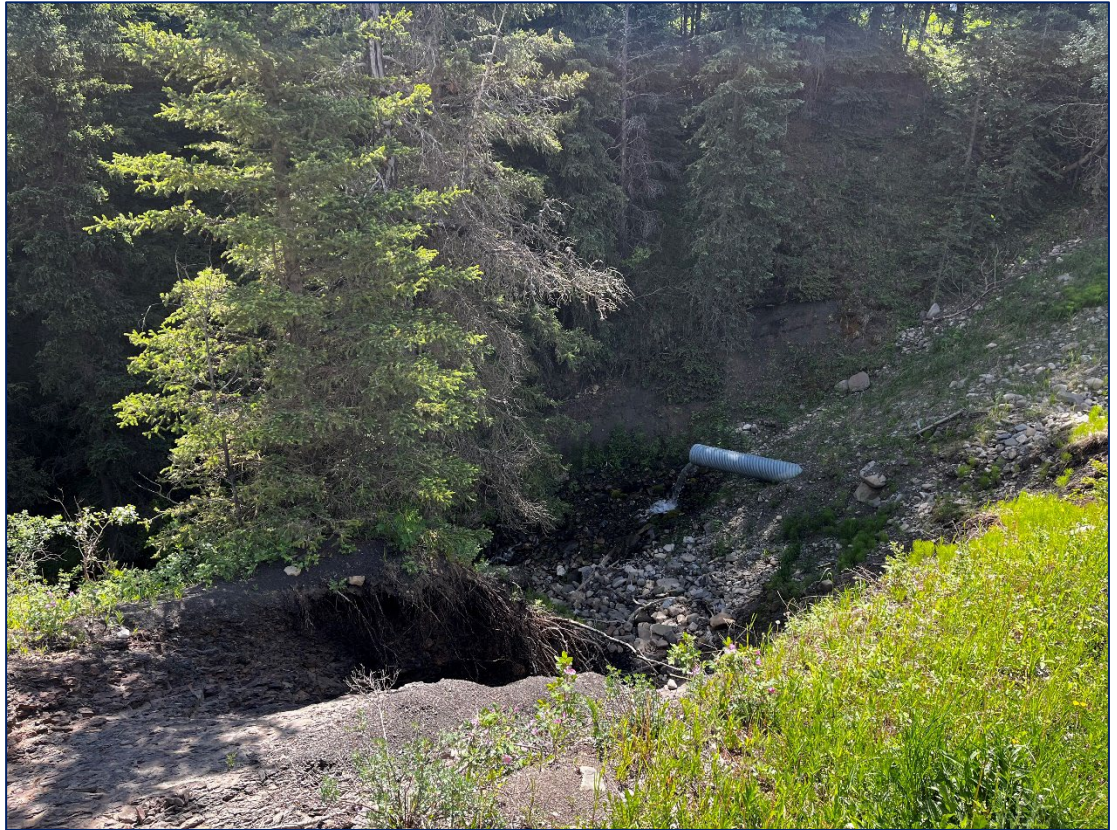
View looking downstream from NE corner of crossing. Severe erosion occurring along embankment and banks of channel.
